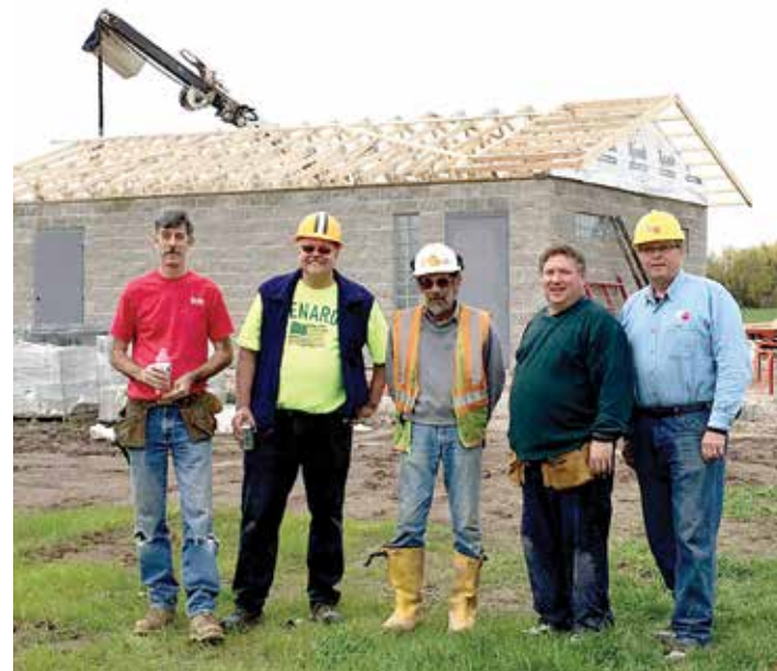
Construction of the concession stand: Russ Reynolds, Marty Briggs, Scott Borkowski, Eric Orfield, Steve Daavettila.
